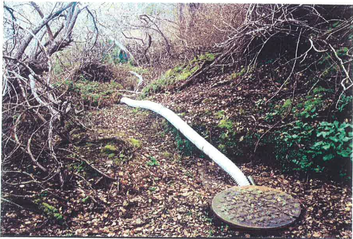
Combined laterals flowing into MH 30
